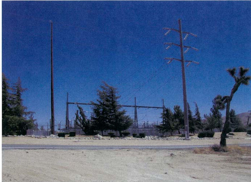
NEC – LOOKING EAST AT SUBSTATION (September 2004)
