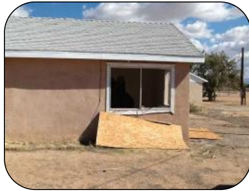
40 Abandoned Unsecured Building Cases
