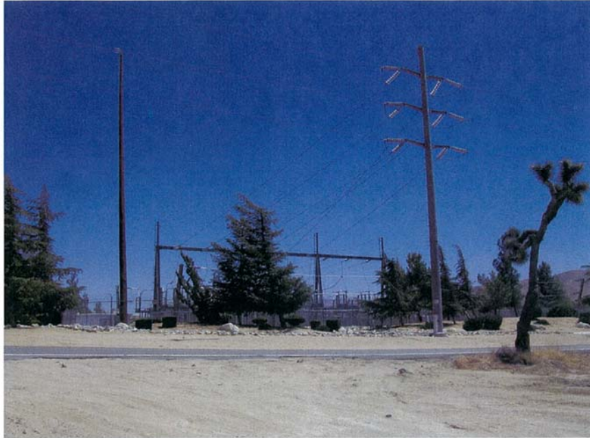
NEC – LOOKING EAST AT SUBSTATION (September 2004)
