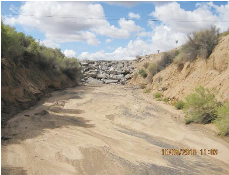
Erosion in ephemeral wash caused by concentrated urban run-off, Hesperia
